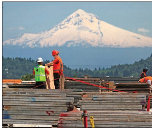
Construction is well underway on the $138 million underground storage reservoir on Powell Butte in Southeast Portland.
